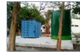
Bio-Gas Plant, 250 kg/day at M/s Timken
