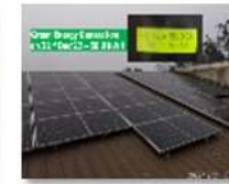
Solar Plant 15 kWp at M/s ZF India
